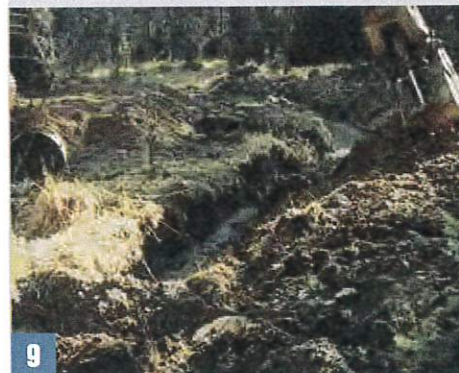
9 After checking to be sure the new culvert is working, close the dewatering channel.
