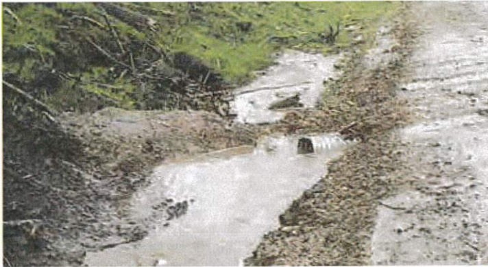
This undersized cross-drain culvert resulted in a breached ditch block and sediment flowing directly into the stream. With proper cross-drains, water cannot soak into the road, causing surface softening and rutting.
