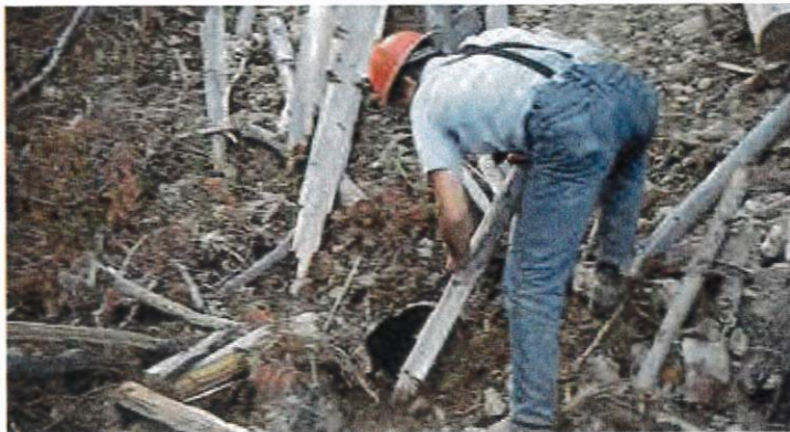
Hand, shovel, and chainsaw work are usually all that culvert maintenance requires. But don't delay! Delay in cleaning a blocked culvert or ditch can result in a damaged road that requires costly reconstruction.
