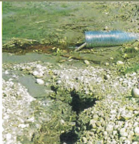
This ditch flowing directly into a stream has resulted in sediment delivery. An additional drain culvert or rolling dip should be installed.
