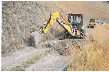
A backhoe is the best choice for open top pipe culvert installation.
