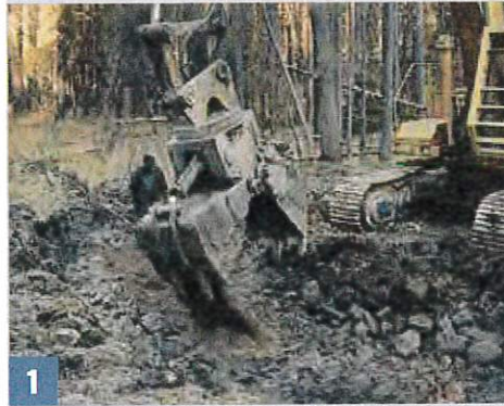
1 Construction of culvert stream crossings has the greatest potential to cause immediate sediment pollution. Installing culverts is more than just placing a pipe in a stream. Complete the work promptly, at a time when the least damage will occur.
