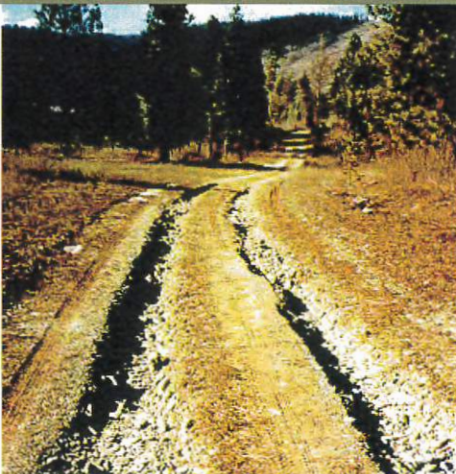
Water runoff formed these long narrow chutes or rills, running down-slope on the surface of this road. It is a source of sediment.
