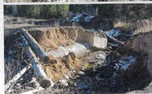
Ignoring BMPs can result in damaged streams, unhappy downstream neighbors, impassible roads, and fines.
