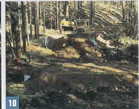
10 The road approach to the new culvert is the next phase of construction.
