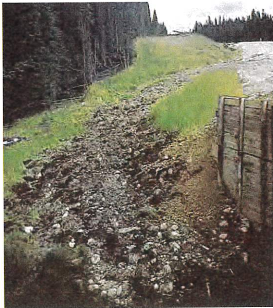
Keep road drainage under control. Sediment is being carried around this bridge abutment and draining directly into the stream.
