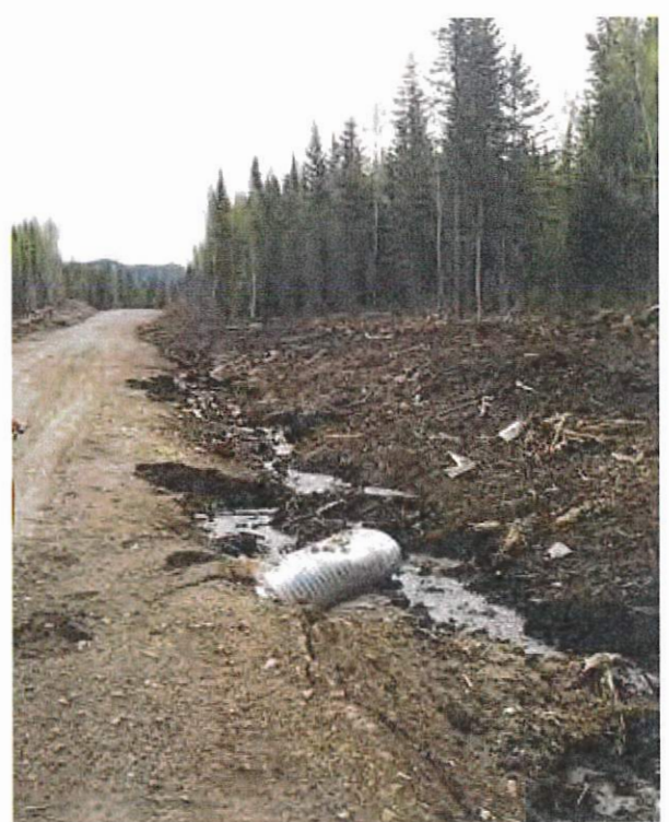
An unusually high flow event contributed to this blown out ditch which resulted in a relief culvert too high to drain under the road surface. A rock armored catch basin at the inlet could have reduced impacts on this site.
