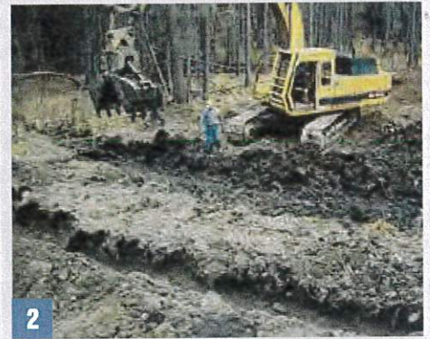
2 The temporary channel in the foreground carries stream water. The dewatered stream channel is being cleared for culvert installation. The channel foundation and trench walls must be free of logs, stumps, limbs, or rocks that could damage the pipe.
